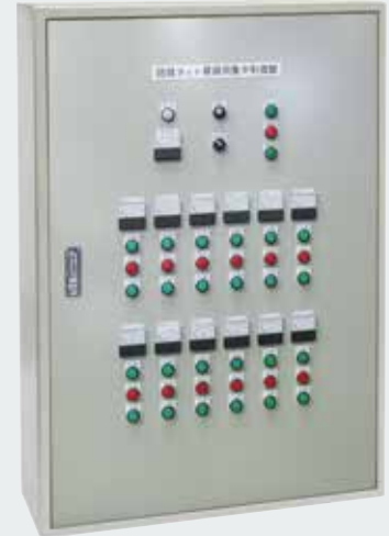
Centralized Control Panel
